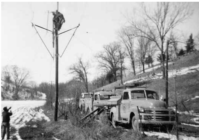
A crew for Grant Electric Cooperative (later merged with Lafayette and Crawford Electric Cooperatives to form Scenic Rivers Energy) works on the lines in 1956. Jim Nodorft says some of the original Grant Electric poles are still standing on his rural Platteville farm.
